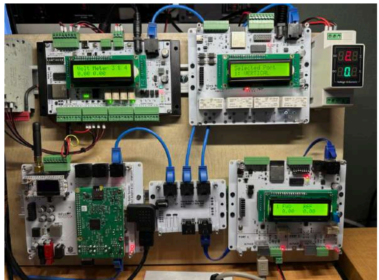
Control Everything in the Shack Remotely
